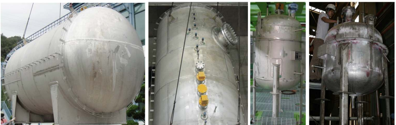
< Sodium Storage Tank >
