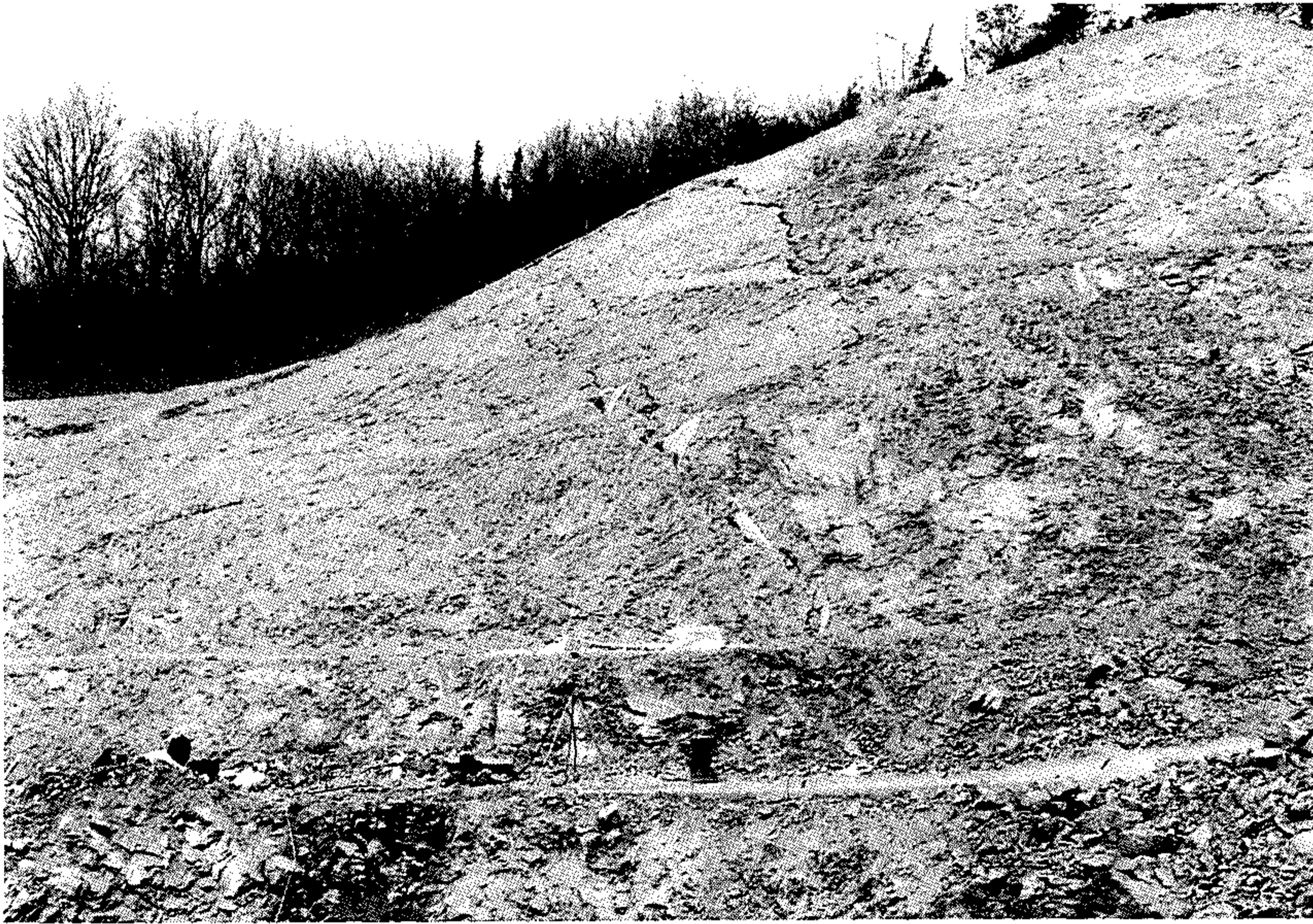
Fig. 41. Example of rock sliding due to the filled discontinuity. Outlook of Pangyo survey area. Severe large cracks in the cut-out area are clearly shown.
