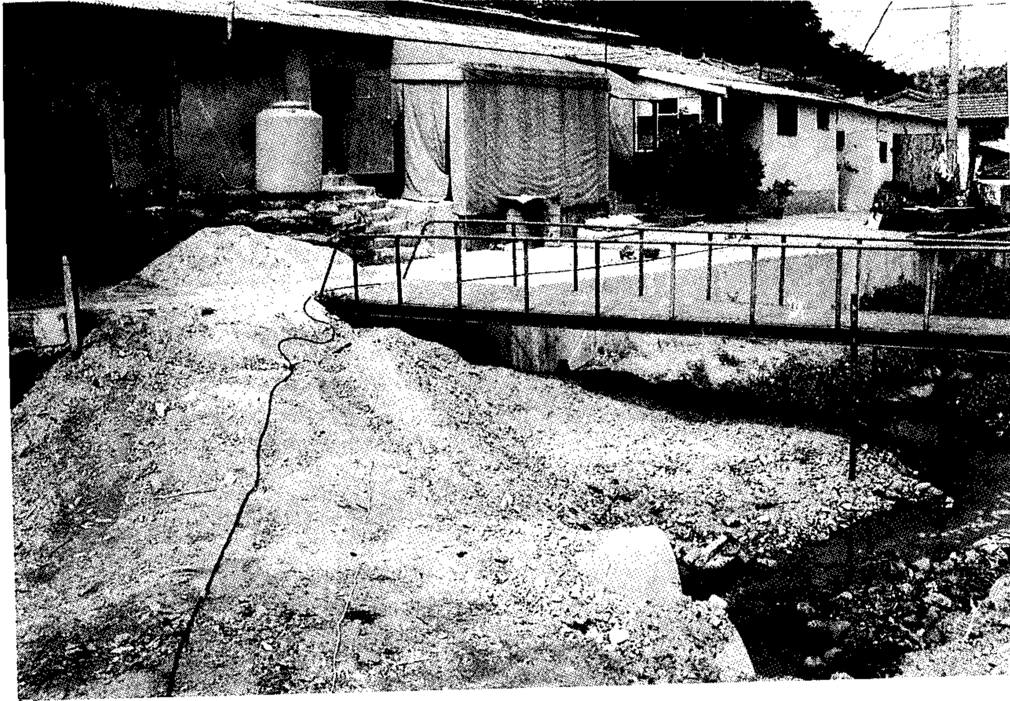
Fig. 52. Subsided area within a streamlet near Bupyong civil cemetery.
